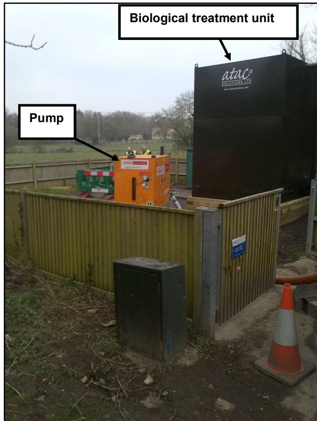
Photo A – Mullen's Pond WPS compound
