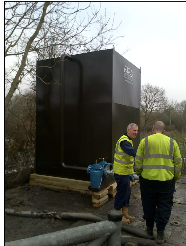
Photo B – Biological treatment unit in compound
